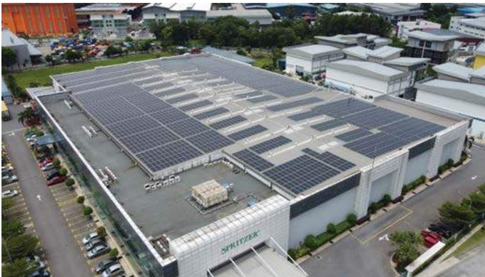
Figure 8 - Rooftop of solar panel installation at Shah Alam plant
